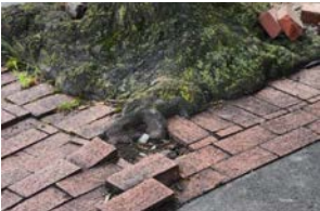
Street trees don't have adequate room and for roots and are pushing up pavement
