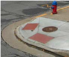
The transition from the curb ramp to the roadbed should be flush, but they degrade making it hard cross the street on wheels
