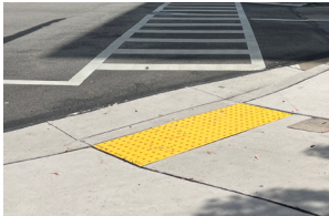
Curb ramps are often too steeply sloped, even the 8.33% code minimum is challenging. They are also often too narrow, which doesn't allow people to cross together.
